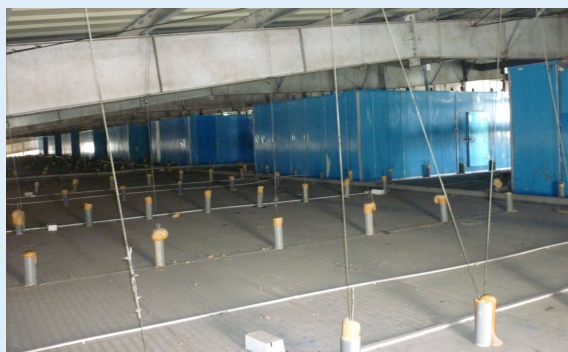
The penthouses are located on the roof of the insulated cold storage facility, underneath the protective pitched roof.
