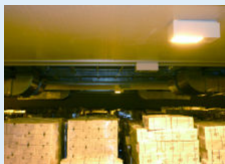
The ducts provide for the necessary air distribution
