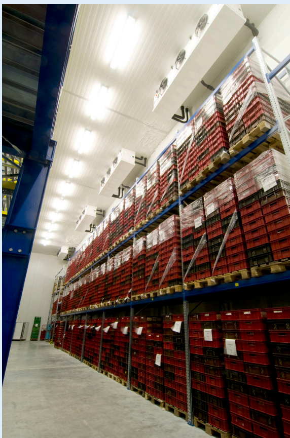
CO 2 evaporators in the deep-freeze room
