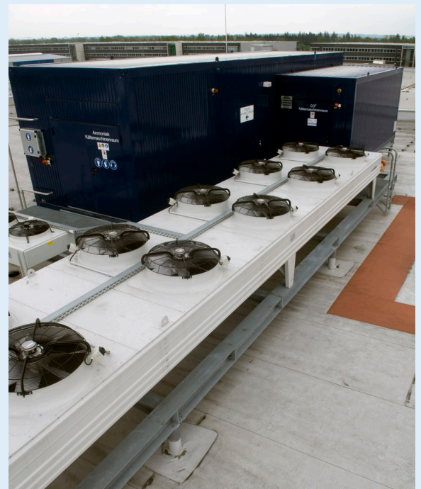
NH 3 condenser AGVH
