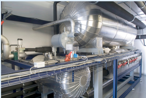
NH 3 /CO 2 machine assembly within the container
