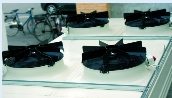
Güntner CO 2 gas cooler/condenser
