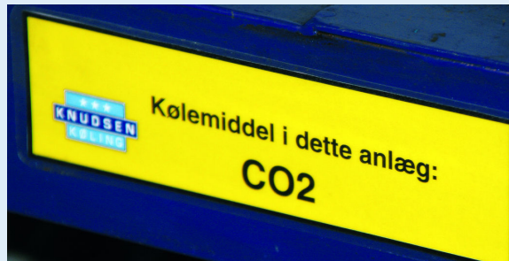
Plant refrigerant: CO 2
