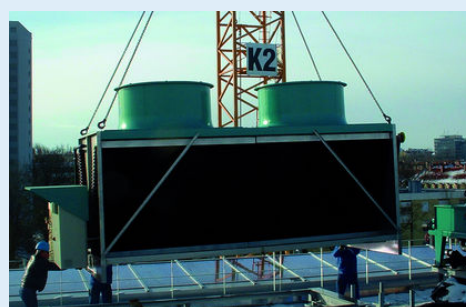
Hybrid coolers of Jäggi/Güntner: Ideal for the application in clinical areas due to the absence of legionella and the emission protection suitable for clinics. Photo above: 2 HTK, model 1.8-52-2S-B6-BU-SX3.
