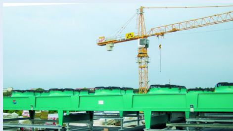
On the rooftop of the RPTC, there are 9 Güntneraxial drycoolers, model S-GFH 102C/2x5-S(D)-F4/2P.
